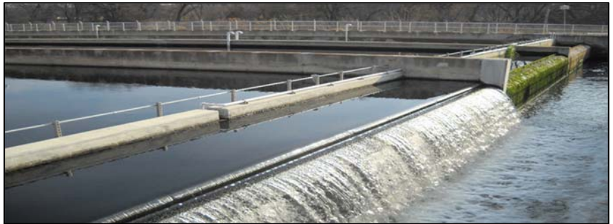
Fox Metro Water Reclamation District wastewater treatment plant
