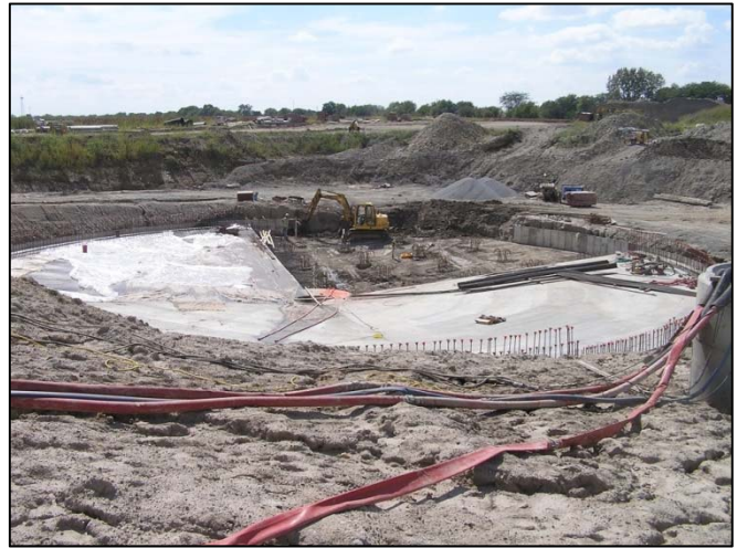
Construction of the base of the 1.5 million gallon first flush tank at the Riley Creek CSO Satellite Treatment Facility in the City of Mattoon
