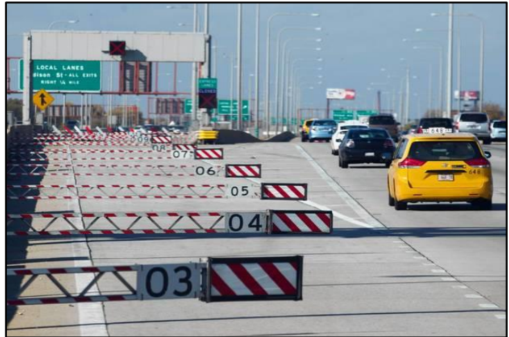
Swing gates on the outbound Kennedy Expressway
