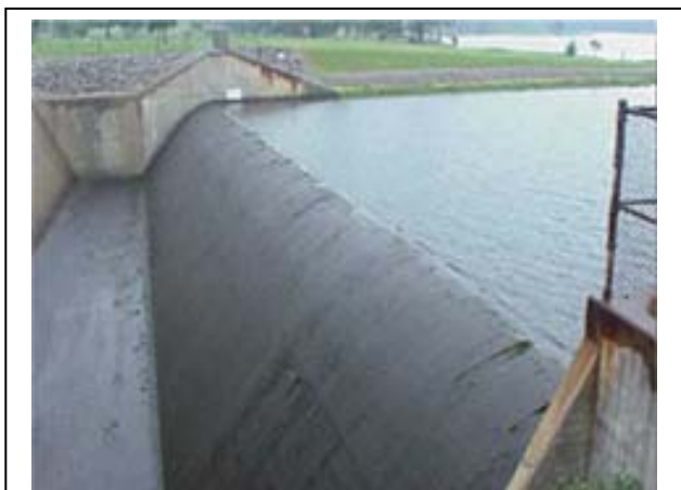
The dam spillway at Lake of Egypt in Williamson County aids in control of the flow of water from the lake.
